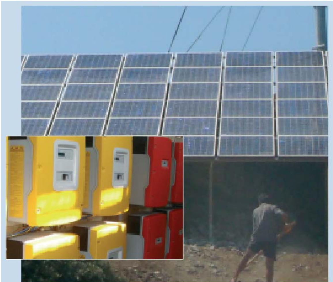
Fig. 5 - PV-wind-diesel generator hybrid power system in an island in Fethiye-MUGLA by Girasolar Ltd.
