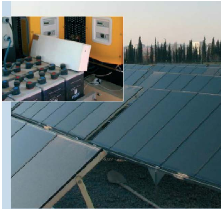
Fig. 8 - HYDEPARK Project in TUBITAK-MRC in Gebze. (12 kWp PV modules, 5 kWp wind turbine, 2,4 kWp PEM type fuel cell, 48 V 1500 Ah battery capacity, inverters, a meteorology station, etc.).
